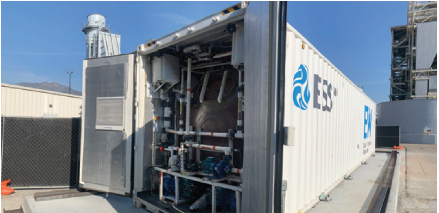
A view of the energy storage unit. Photo courtesy Burbank Water and Power, California
